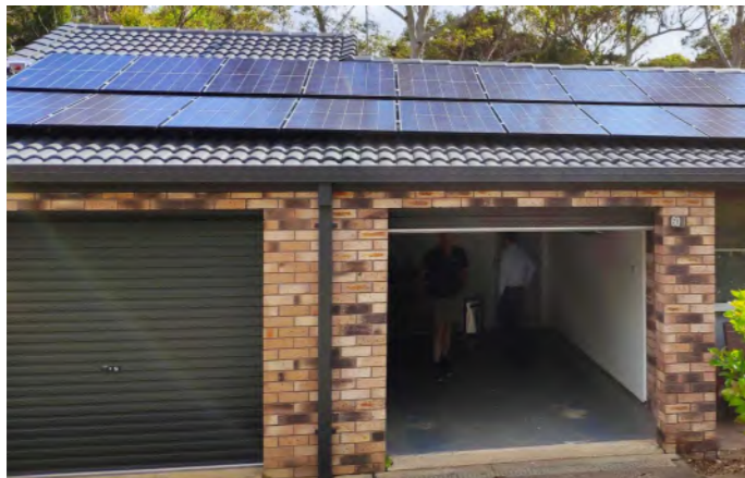
Australia, Melbourne 6kW, Growatt SPH6000
